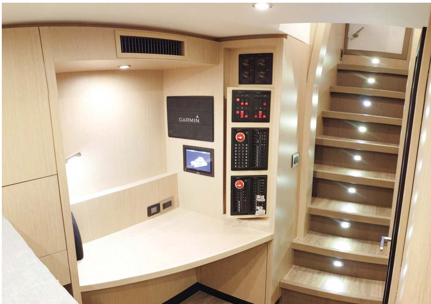
Desk Area with Master Control Panel and C-Zone Digital Switching System.
